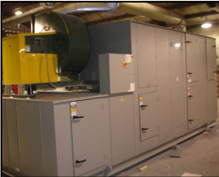
The unit, ready to be shipped.
