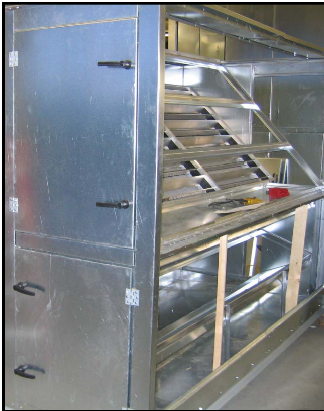
With End Panels Removed, the Face-and-Bypass Damper behind the Filter Rack is visible.
